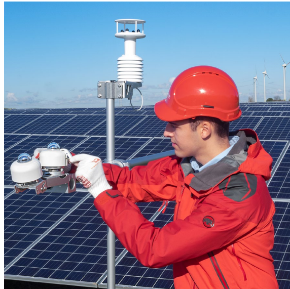
Figure 0.3 SR30 includes a digital tilt angle measurement, very practical for remote checks of instrument orientation. The image shows two SR30's in PV system monitoring, one measuring in Plane of Array (POA).
