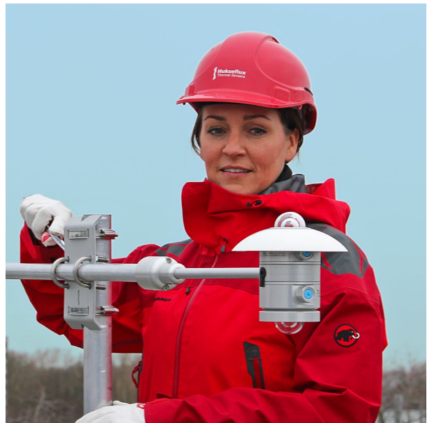
Figure 6 Installation of AMF02 albedometer mounting kit and two SR20 pyranometers, mounted with ALF01 levelling fixture on a crossarm with crossarm bracket CMF01.
