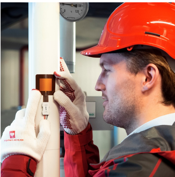
Figure 2 FHF04 being installed to measure heat flux on a pipe
